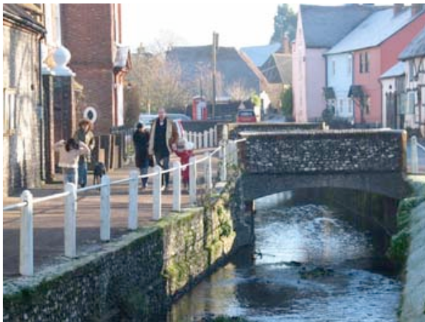
One of the six bridges which span the river during its course through East Meon
