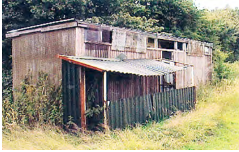
The soccer changing rooms – a dilapidated animal shelter
