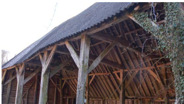
Fig 45 Lythe House barn, with aisle on far side; slots on the outside of near-side posts indicate that there was originally a second aisle
