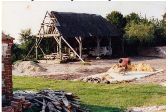
Four of the five bays of the barn, new farmyard entrance to the south.
