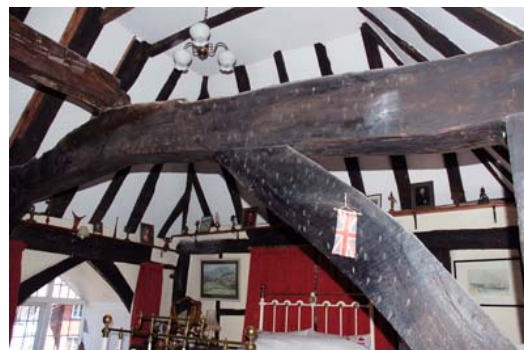
Fig 13 Smoke-blackened beams in what is now the upper floor
