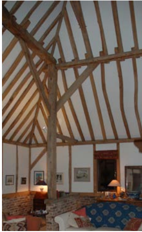
Fig 39 (left) Post and up- braces in today's sitting room, with tie beam and purlin
