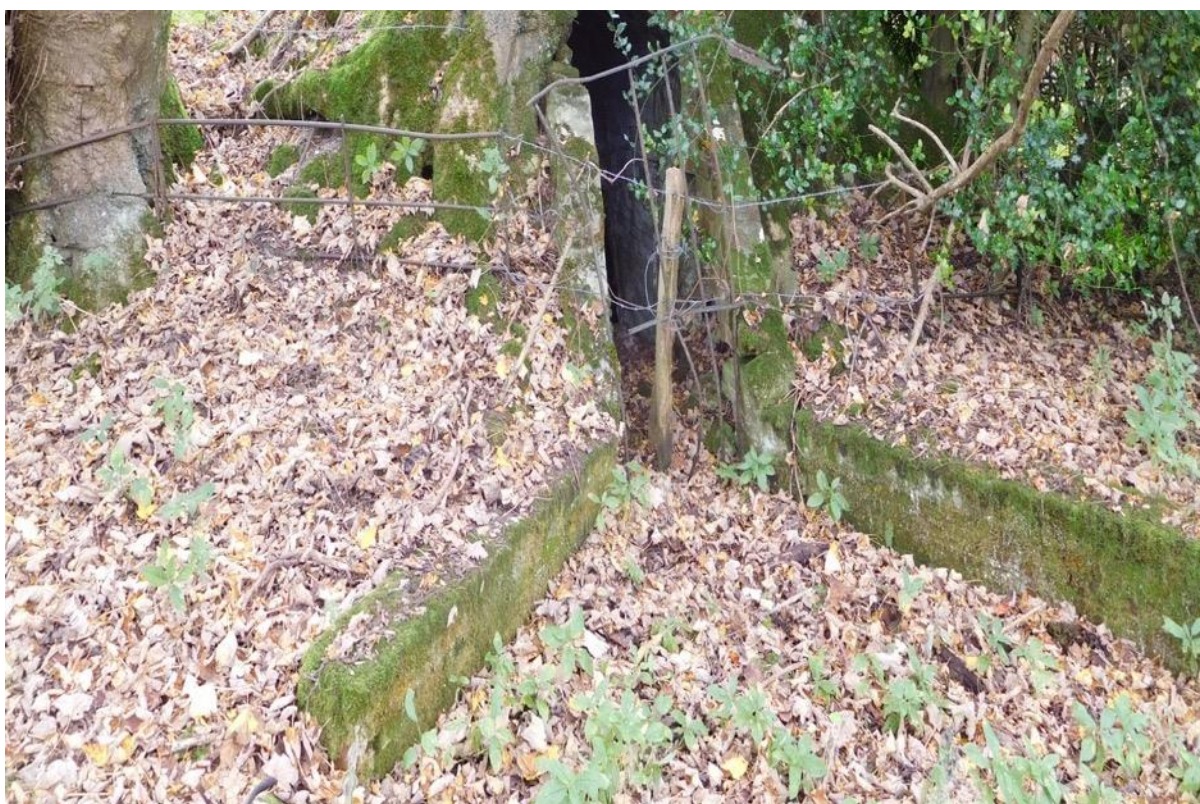
Figure 20: The roots of mature trees are beginning to significantly impact on the structure of the ice houses
