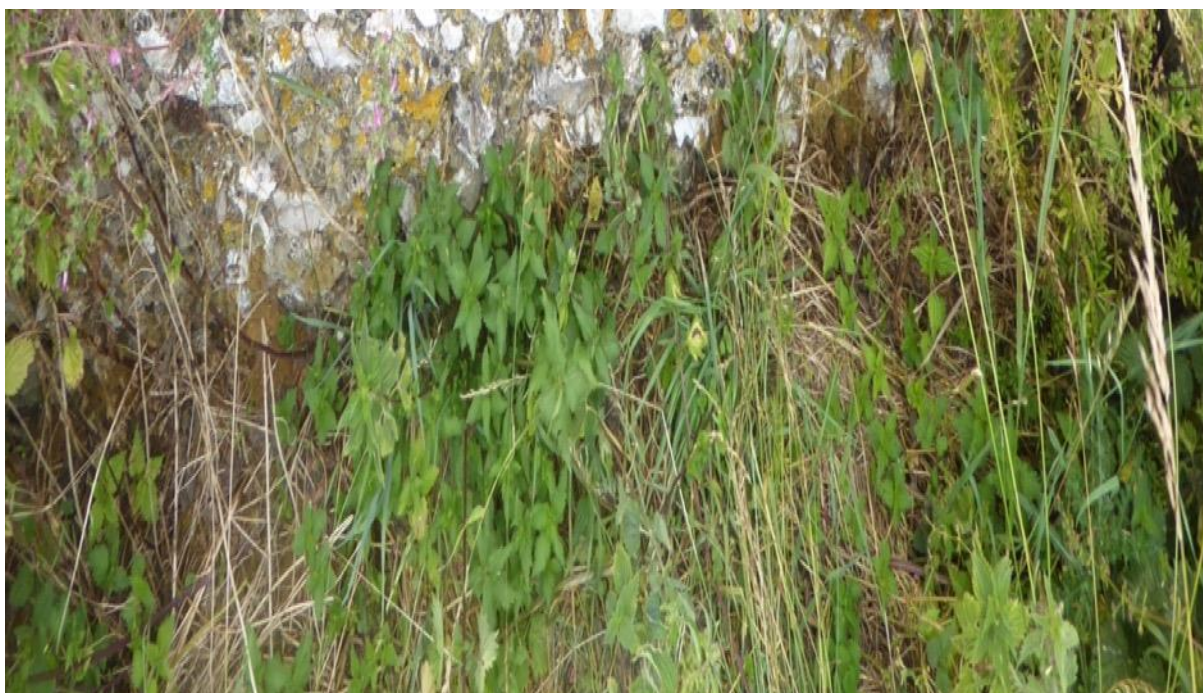
Figure 24: Retaining flint wall element of the 18 th century Ha-Ha to the south of the house
