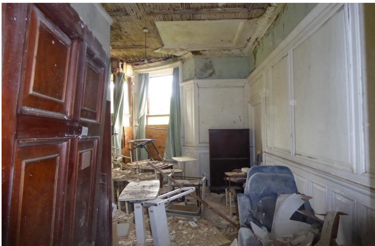
Figure 12: Plasterwork and panelling surviving albeit in a very poor condition
