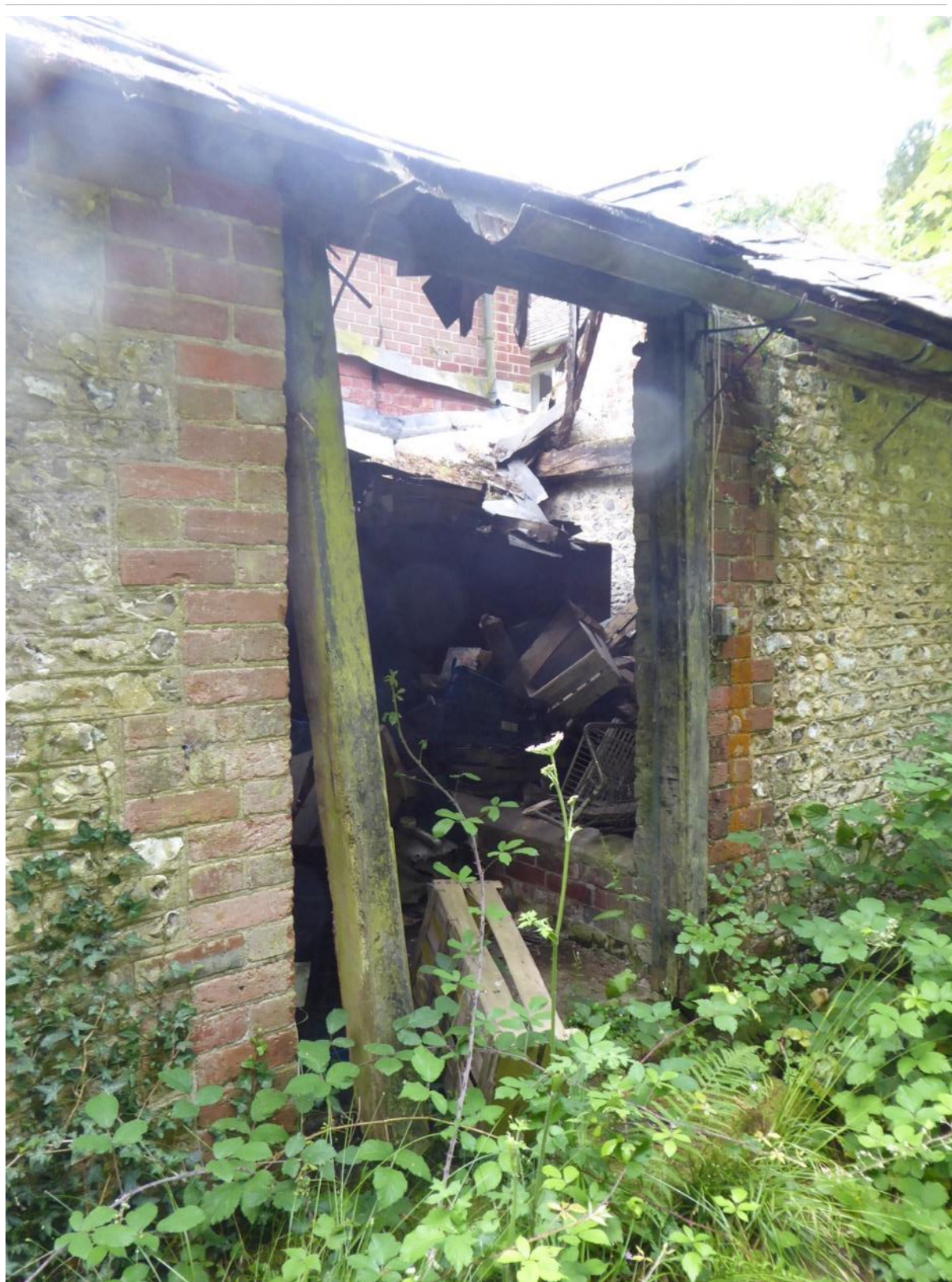
Figure 10: Partially collapsed roof of former 'boiler house' (to east of Westbury House)
